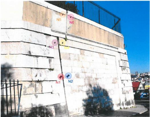
Figure 5.2. Position of the topographical marks of the East wall (Teixeira Duarte, S.A., 2017a)
