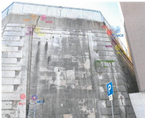
Figure 5.3. Position of the topographical marks of the North wall (Teixeira Duarte, S.A., 2017a)
